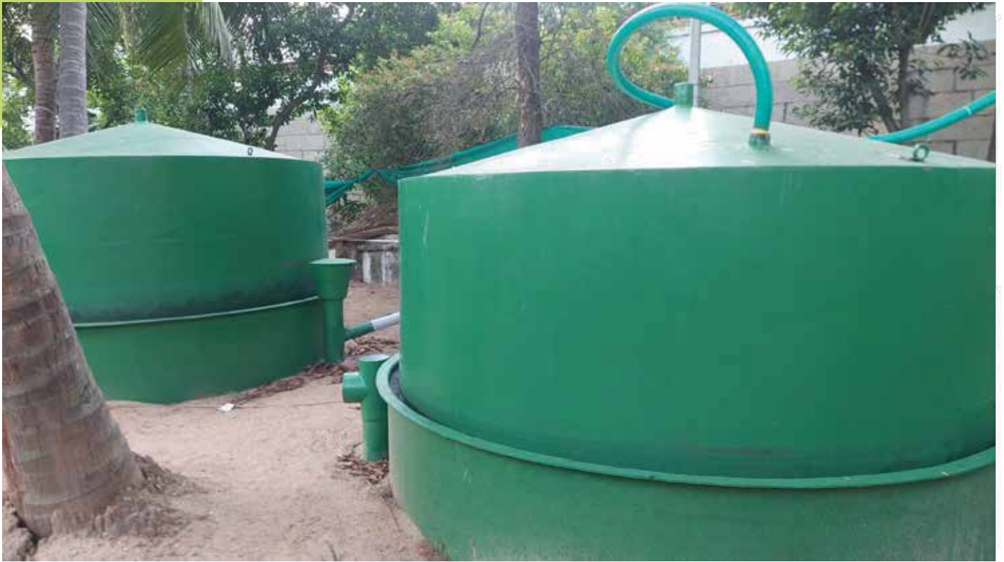
1000kg Biogas plant - Padaleeswarar temple, Cuddalore
