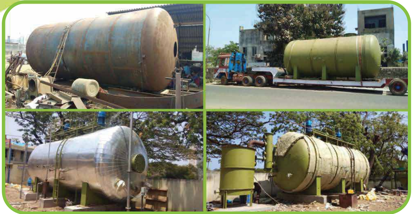
1 TPD - Biogas Plant
