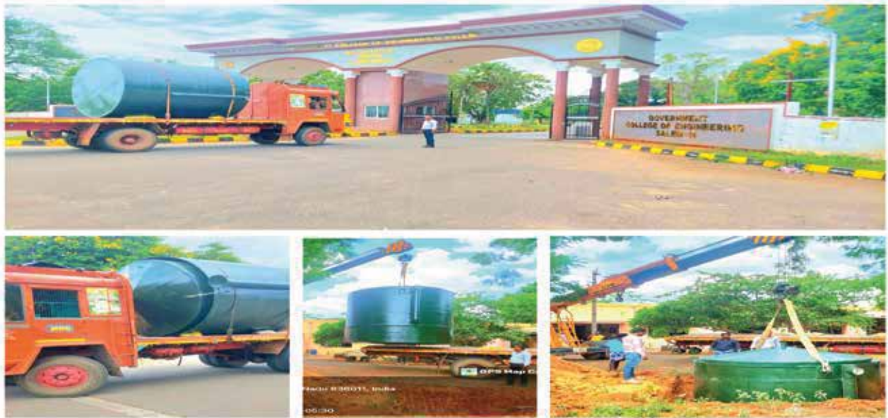
150Kg/Day Biogas plant - Govt.College of Engg, Salem
